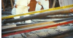
Asbestos contamination of collections and facility.
