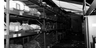
Interior view of Building 26 with contaminated collections and part of the roof missing.
