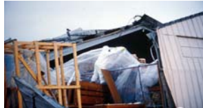
Workers covering collections with plastic for temporary protection until a temporary roof is built.
