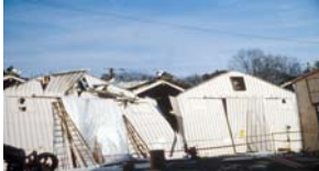
Damage to Building 26 immediately after the tornado.
