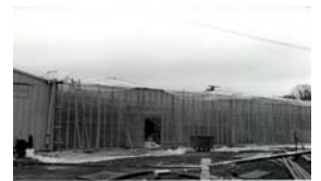
A wood and plastic super-structure is built around the damaged areas of the building to contain asbestos contamination.
