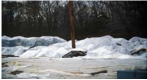
Area surrounding Building 26 draped with plastic to contain debris from further spreading until abatement could begin.
