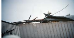
Roof damage at Building 26.
