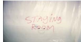
Containment areas and decontamination zones were created inside the building using polyethylene sheeting.
